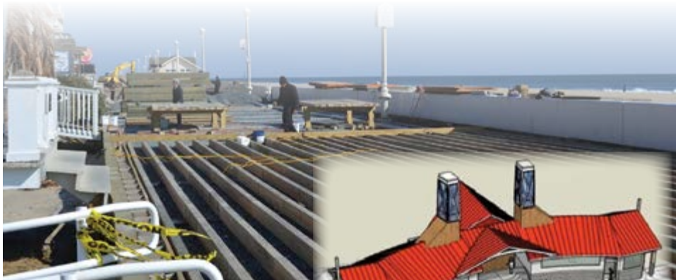
Pictured above the Boardwalk reconstruction At right is a rendering of the Caroline St. building
